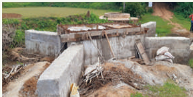
Culvert Construction at Tentuli VSS of Angul Division through convergence with RD Dept.
