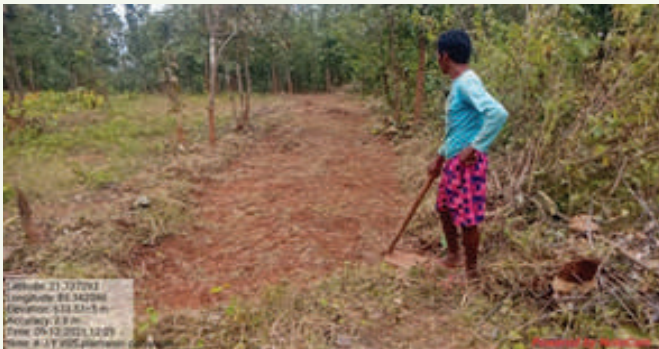
Fire Line creation work at Panasuan ANR plantation site in BJP FMU of Keonjhar Division
