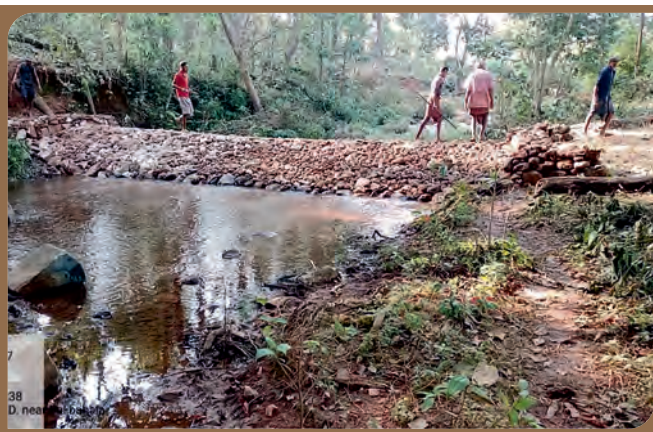
LBCD at Balibahal VSS, Deogarh Division
